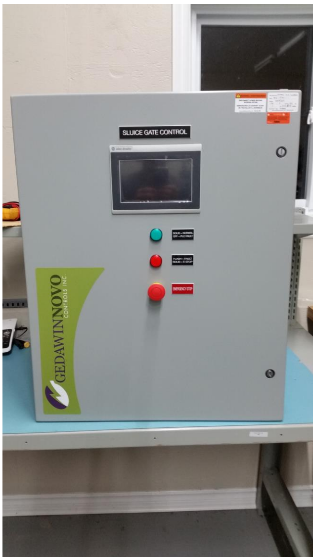
Sluice gate control cabinet
