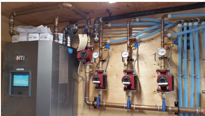
Boiler and pumps for 3 heating zones in gate
